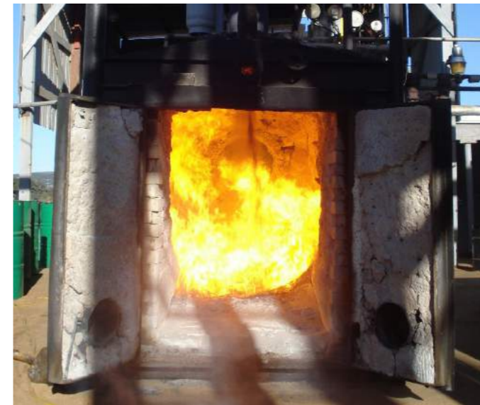
TEXAROME WASTE WOOD BURNING FURNACE for steam production
