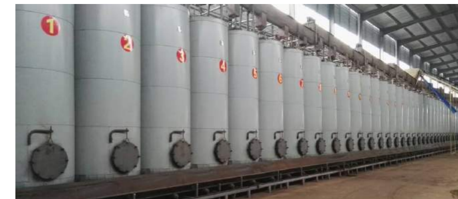
DISTILLATION EQUIPMENT for crude oil from sawdust
