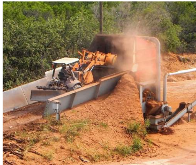
450 HP WOOD GRINDING SYSTEM Texas
